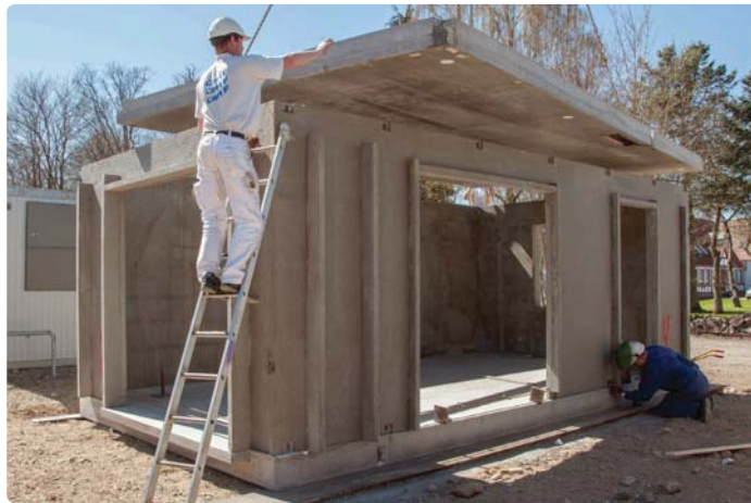
Fitting the ceiling slab onto the assembled walls completes the assembly of the bPod. Steel inserts are used to weld the ceiling to the walls and internal completion and decoration follows before transport to the building site.
