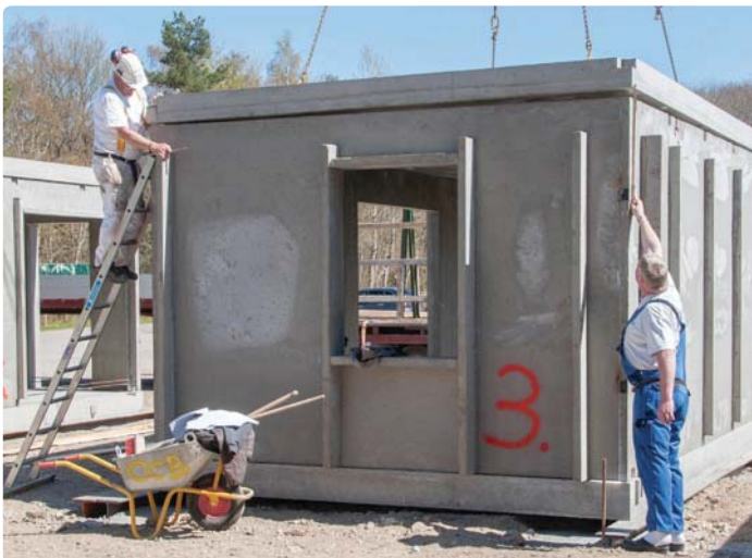
The completed bPod will not be lifted by its ceiling but by chains connected to the floor slab. The assembly of these test pods takes place outdoors while a production line is being prepared. Production bPods will be assembled and finished indoors.
