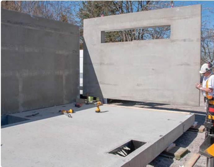
A short wall with an opening for a narrow, horizontal window is positioned in a bedroom bPod. The window will in most cases be installed in the façade elements, which will be added to the assembled bPods on-site.
